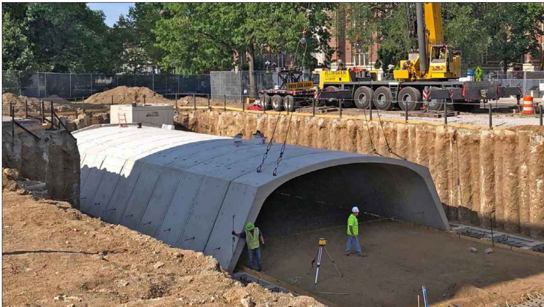
Figure 46. Underground stormwater basin in front of the University of Michigan Museum of Art
